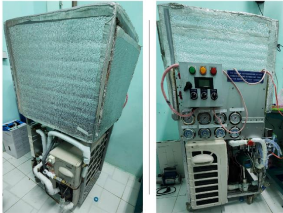
Fig. 2: Photos of R513A/R744 cascade system
