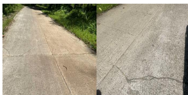
Figure 7. Sample photos of physical damage in the surveyed FMR
