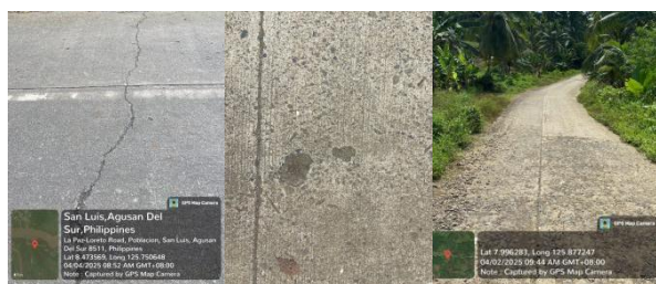
Fig. 4. Observed road damages in various barangays: (a) crack in Brgy. Poblacion, San Luis; (b) potholes in Brgy.
