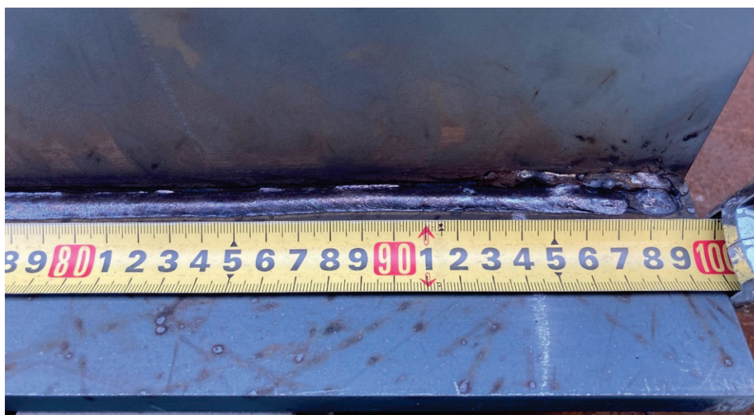
Fig. 5-10 Photograph of weld bead appearance of derailment
