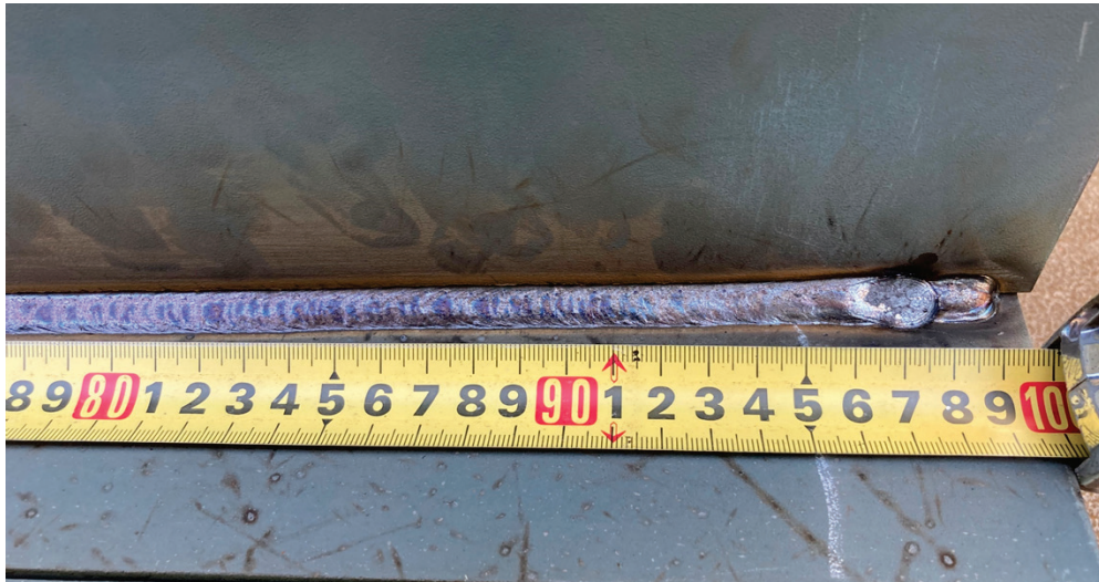
Fig. 5-7 Photograph of weld bead appearance of normal condition
