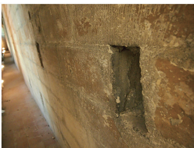
Fig. 15. Saint-Leu-d'Esserent, priory church. Putlog holes
