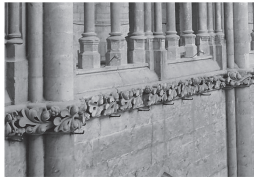
Fig.3 Amiens Cathedral, nave. Iron hooks under the foliage frieze of the triforium.
