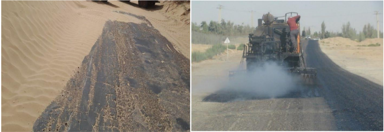
Figure. 2.6. Asphalt Surface Weathered by Dust Storm (Miri & Middleton. 2022).
