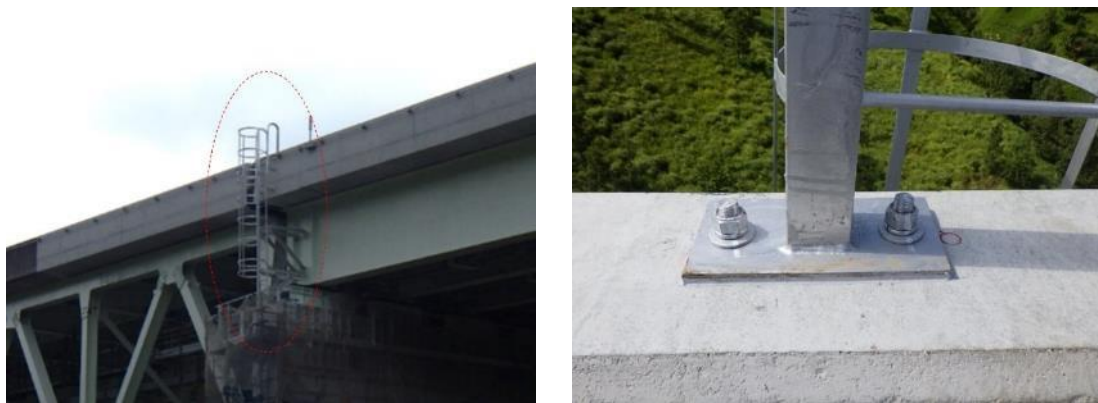
(a) The ladder coated by hot-dip Al coating (b) Hot-dip Al coated steel plate contact with concrete
