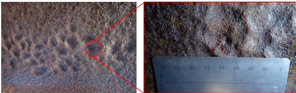
Figure 5-1 Extensive pitting corrosion on a weathering steel bridge member.
