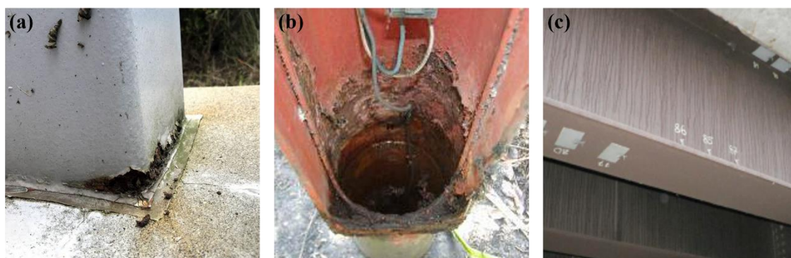
Figure 1- 1 Representative atmospheric corrosion locations of steel members including: (a) steel members in boundary with ground[13], (b) enclosed sections [14], (c) high-humidity areas[15].
