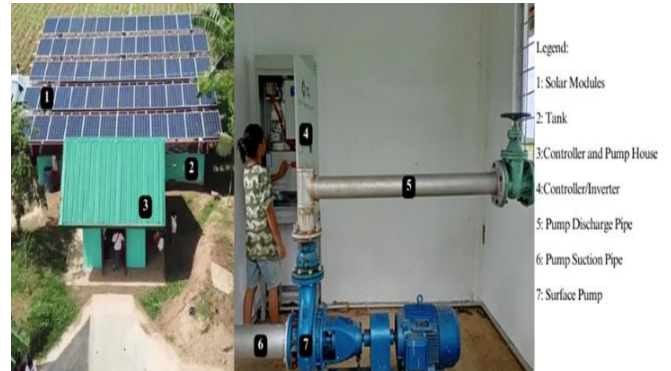
Fig. 3. Components of the SPIS installed at Brgy. Pag-asa, Sta. Josefa, Agusan del Sur.
