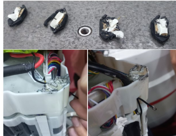
Fig. 13. Severe Damage to 4 Elastic Foundations and Damage to the BMS Holder
