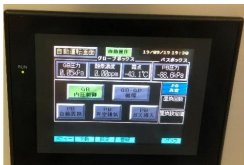
Figure 51: passing box control panel.
