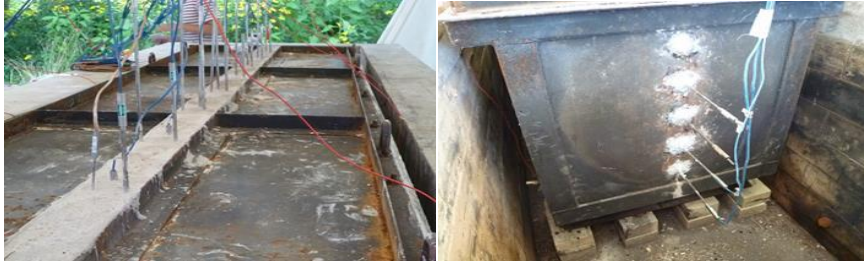
Fig. 7. The temperature sensor buried above and to the sides of the steel container
