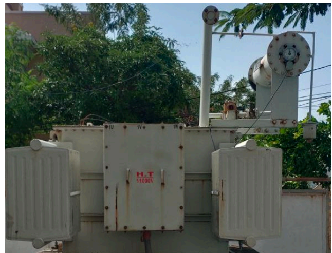
Figure 2 Heavy duty transformer at company site (Jaipur)
