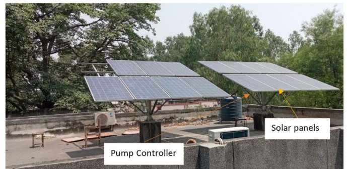
Fig. 9: solar panels arrangement
