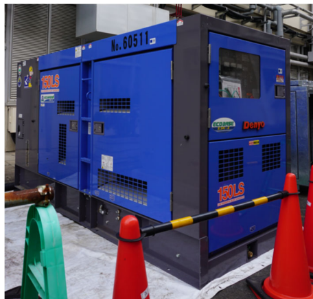
Fig. 4.3 125-kVA diesel synchronous generator
