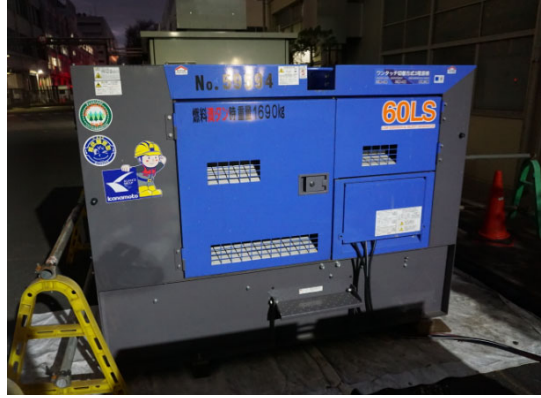
Fig. 3.10 50kVA diesel synchronous generator outdoor
