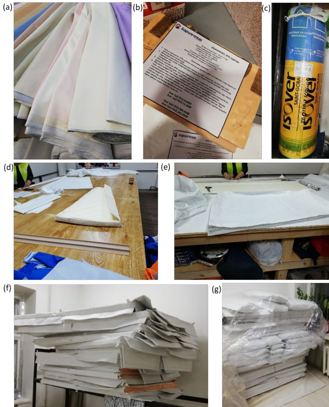
Fig. 3.12 Local materials and manufacturing process: (a) Wall cover fabric; (b) Extruded polystyrene foam insulation board for wall panels; (c) Mineral wool for roof panel; (d) (e) Local manufacturing process; (f), (g) Final locally manufactured panels
