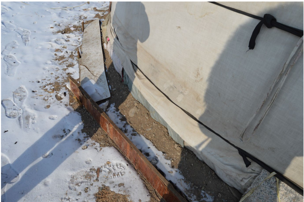
Fig. 2.15 External view of the joint between the wall and the floor of a ger
