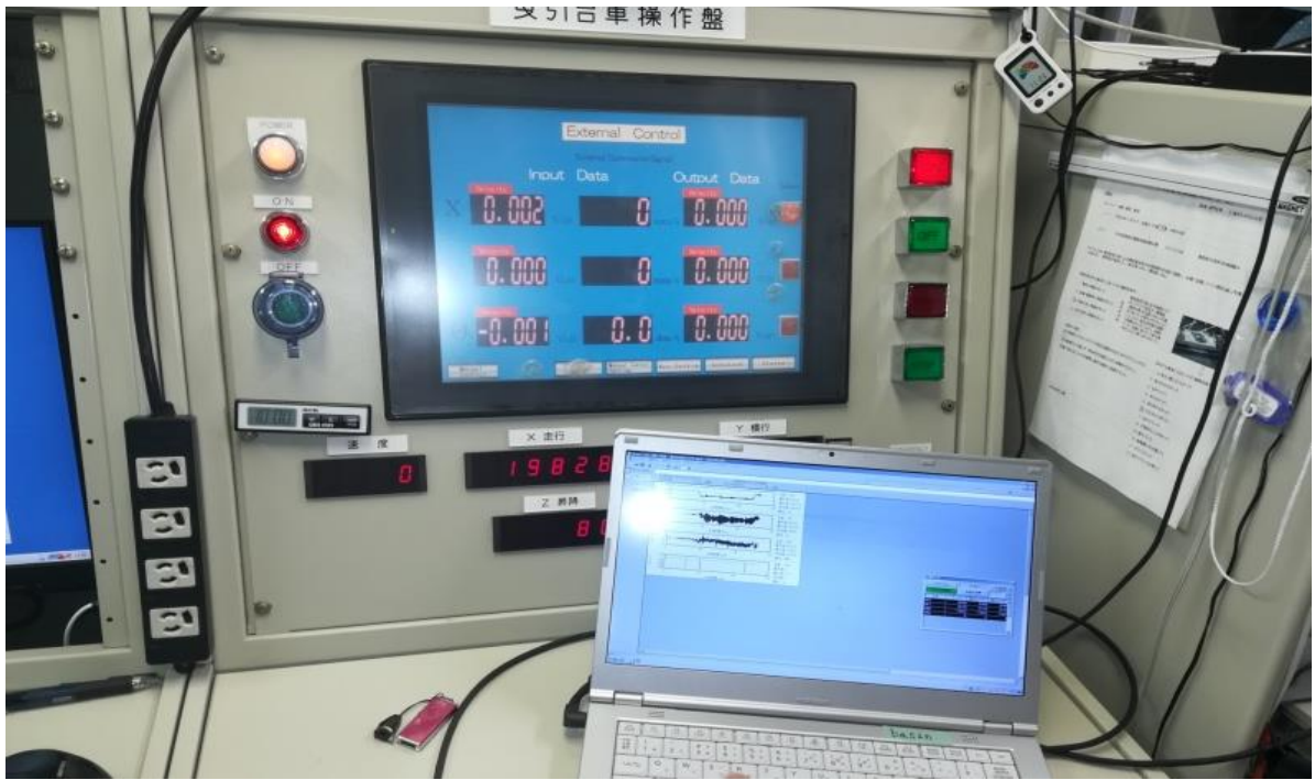
Figure 4-8 CPCM Control Room
