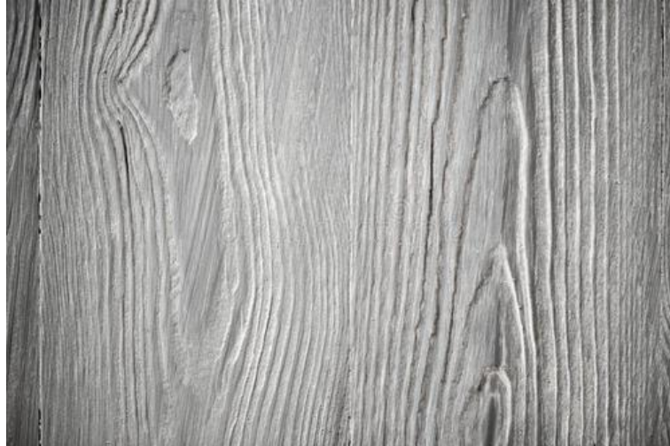
Figure 2.2 The corrugated appearance of wood after weathering.
