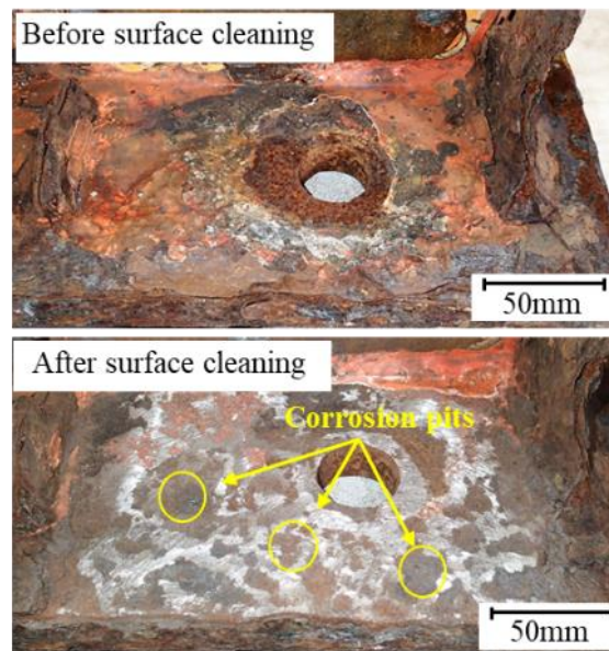
Figure 3-3. Surface conditions of severely corroded steel member before and after removing the rust layer.
