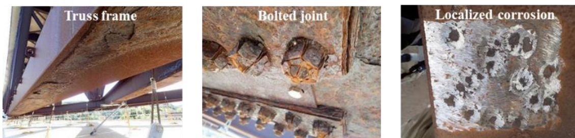
Figure 1-2 Corrosion problem of weathering steel bridge.
