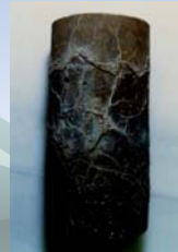
Deterioration found in PARI, in marine tidal condition
