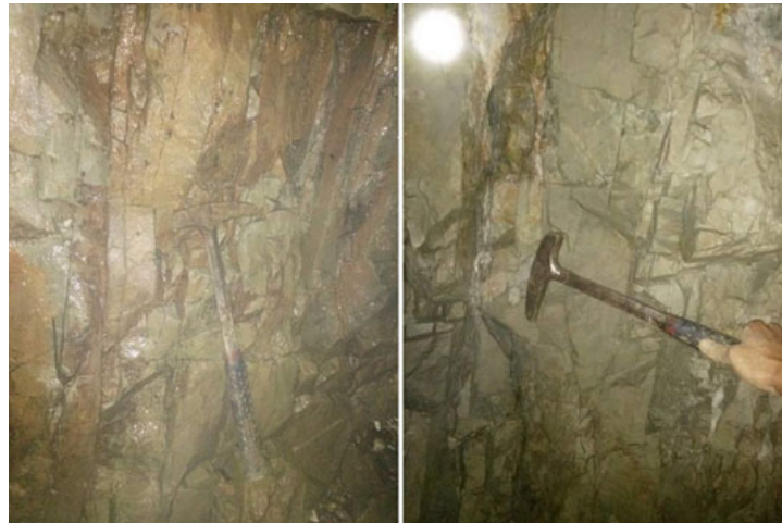
Fig. 5. Rock mass condition in underground tunnel showing joints and cracks.
