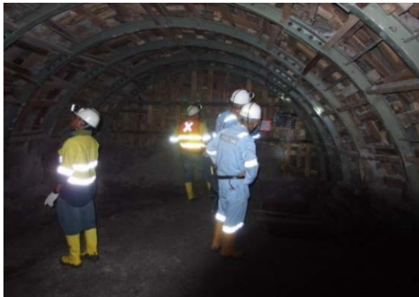
Fig. 11 Steel arch support.
