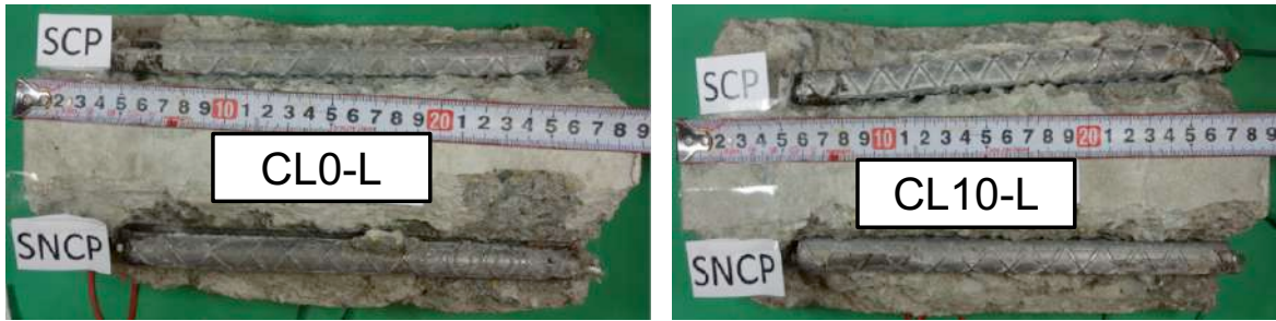
Figure 3.46 Appearance of rebar corroded area in CL0-L and CL10-L
