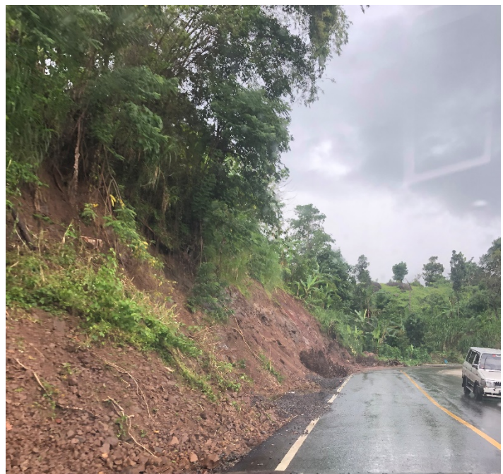
Figure 36 Shallow landslide along the road (January 30, P. Nurdin).
