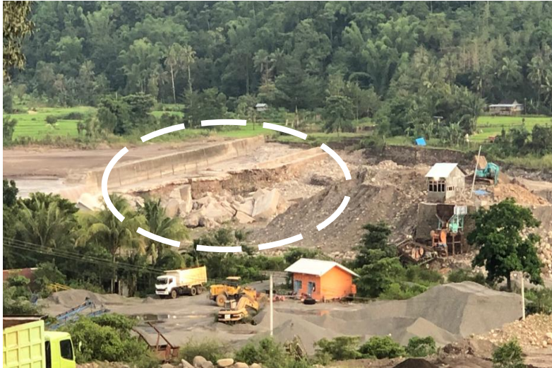
Figure 32 Damaged sand pocket (January 30, A. Soma).
