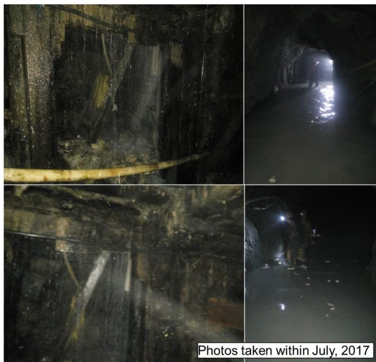
Figure 2.12 Underground adits condition seeping with meteoric water.
