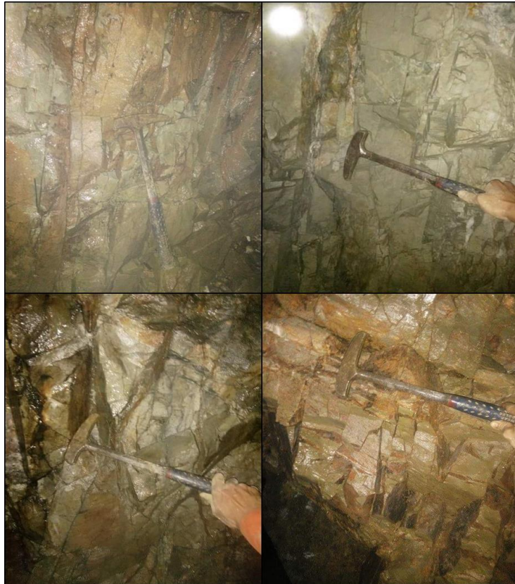
Figure 2.11 Rock mass condition showing joints and cracks.
