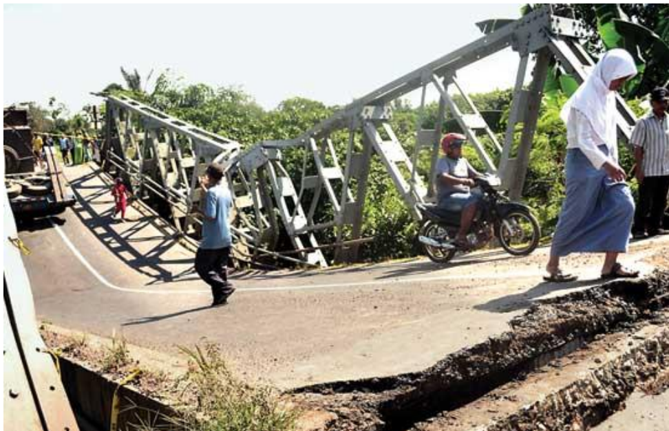
Figure 1-1 Condition of a bridge in Indonesia
