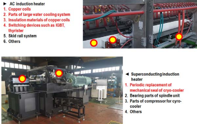
Fig. 1.19 A comparison of major maintenance components between SIH and a conventional induction heater
