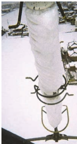
(a) I-arranged suspension long-rod insulator set
