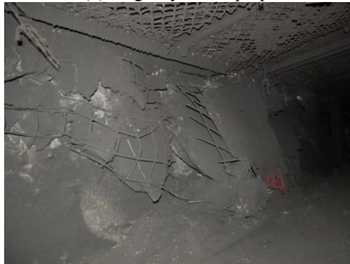
(f) Packfillings collapse
