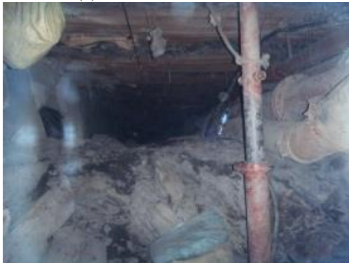
(e) Floor heaving
