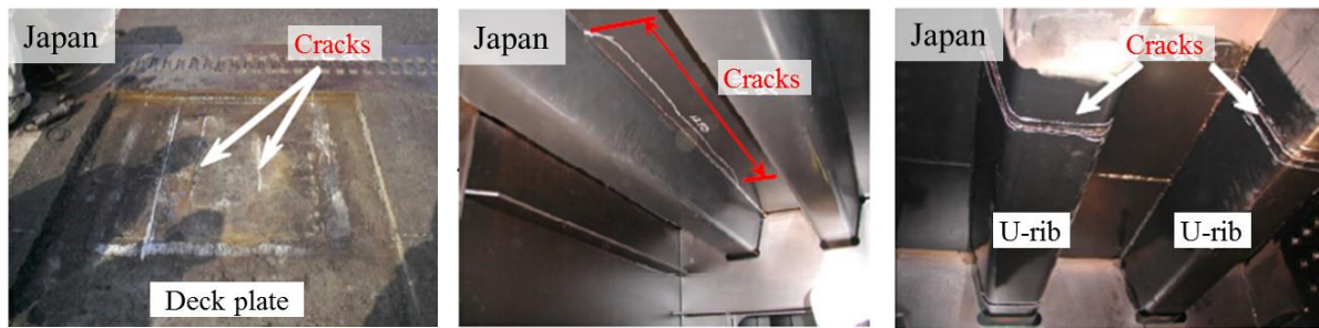
(a) Root-deck crack
