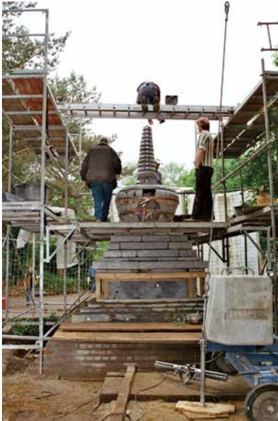
Figure 7. Construction of the stupa in the Rhododendron Park in Bremen, Germany. Photograph by Olaf Hudecek, 2003.
