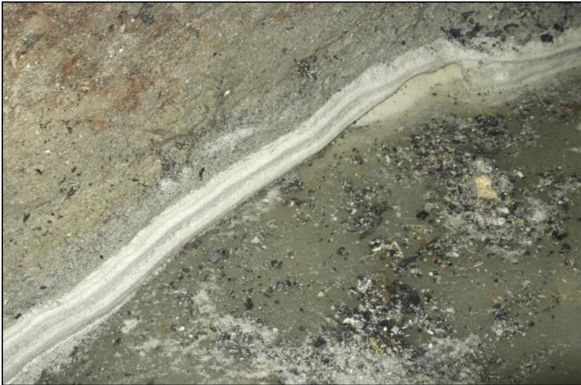
Figure 5.4 Accumulation of calcite scum on the side-wall of the quenching tank in the real incineration facility. The width of the calcite band shown in the photograph is around 5 cm.
