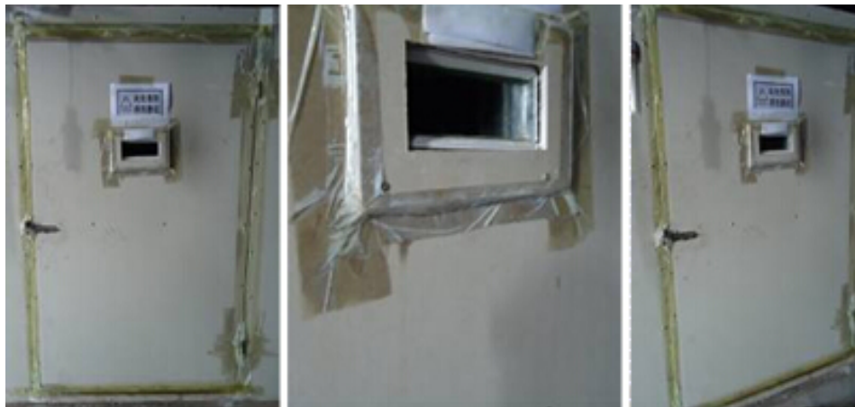
Figure 4-15 Water condensation observed on the window
