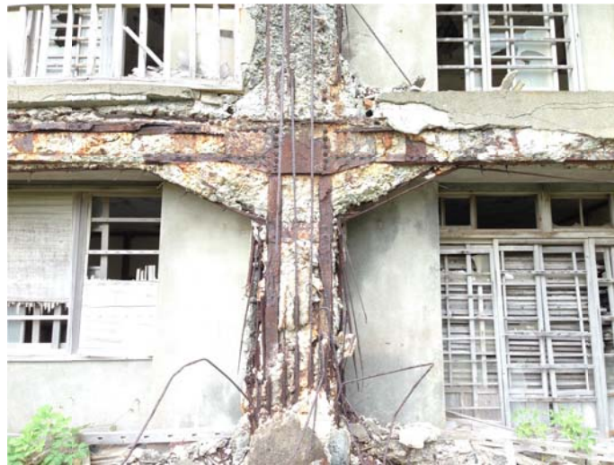
Fig. 2.1 Cracking, spalling and loss of bond between steel and concrete due to corrosion
