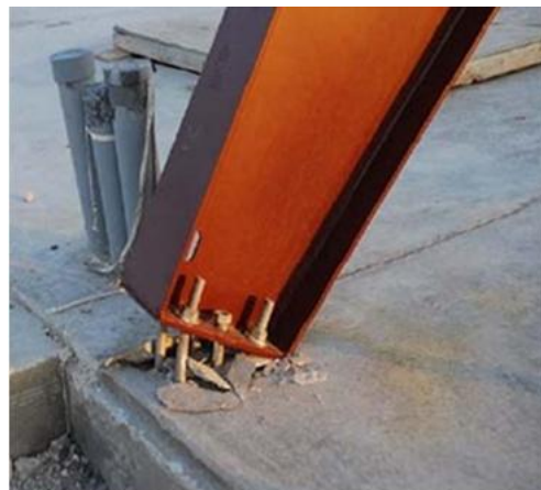
(b) Base plate of column ( https://www.osha.gov/doc/engineering/2012_r_04.html )
