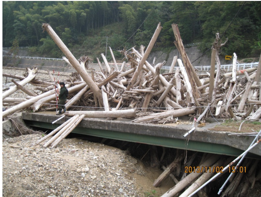
Figure 1.3 A bridge blockage by woody debris in the Nayoshi River, Tsuwano Town, Shimane prefecture, Japan during the 2013 flood.
