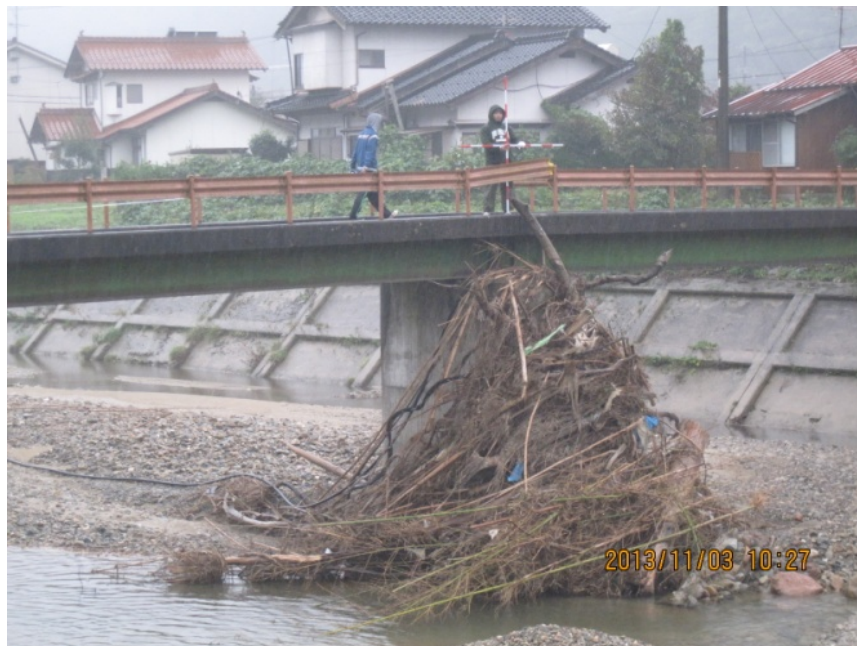
Figure 5.2 A woody debris jam formed by a bridge with a pier in Tsuwano Town.
