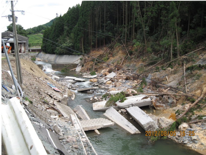
Figure 2.1 A side erosion along the upstream river reach in the mountain area.
