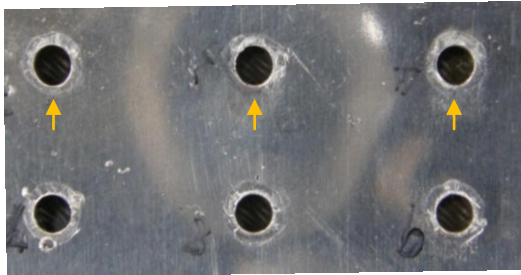
(h) bearing deformation of Al-patch fastener holes (c)
