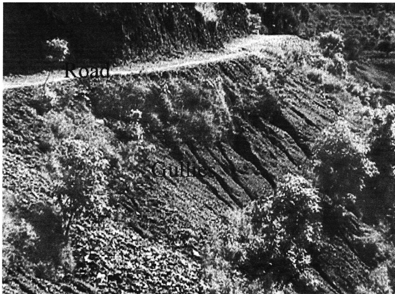
Photo. 2. V shape gully formation on filled bank slope formation below the road.
