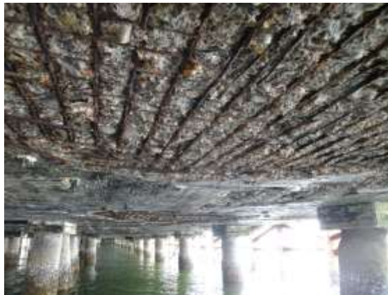
Photo 2.2 Chloride-induced corrosion in a marine environment
