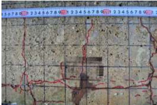
Photo 8.10 Cracks trajectory of L-type beam around center line area
