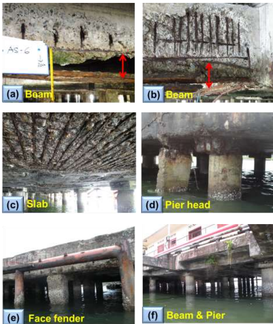
Photo 3.7 Typical deterioration of point B after 77 years of exposure
