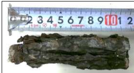
Photo 3.14 Deteriorated steel in concrete
