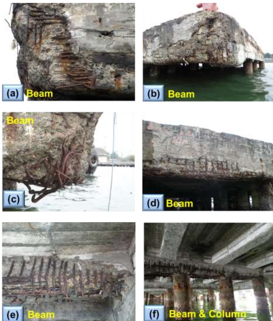
Photo 3.6 Port damages at area A after 77 years of exposure
