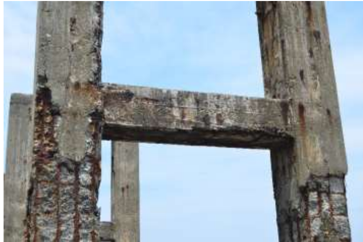
Photo 2.1 Deterioration in a reinforced concrete column
