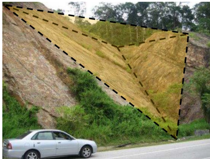
Figure 3.1 The failure wedge by the road.
